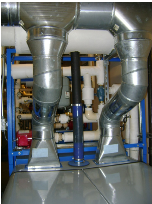
Figure 2. Exhaust Breaching at Engine (CHP #1 as typ) – no test port found
