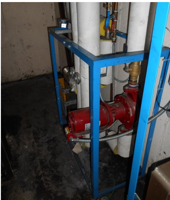
Dump Load Skid
