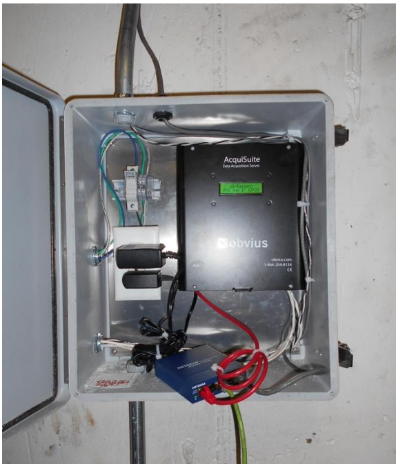
CDH Monitoring Enclosure w/ Obvius Data Logger
