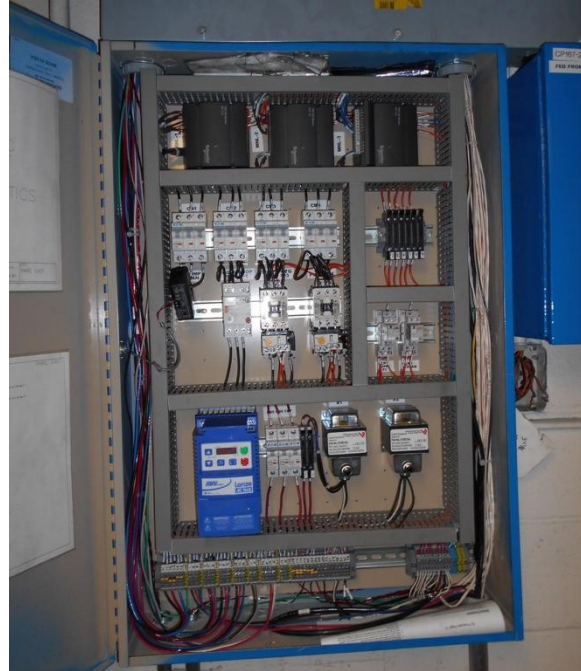
CCP Panel with VFD and Veris H921 Analog CT
