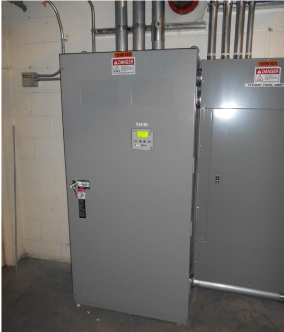
Automatic Transfer Switch and Standby Panel
