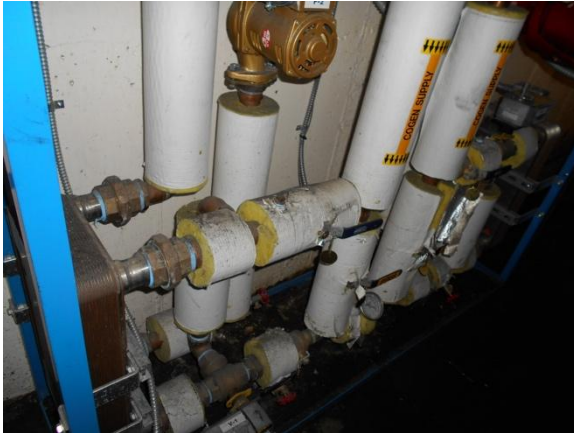
DHW Load & Building Heat Load Skid
