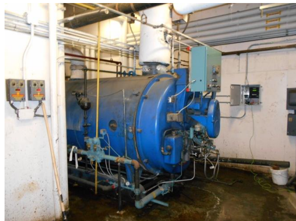
CDH Panel and Existing Boiler
