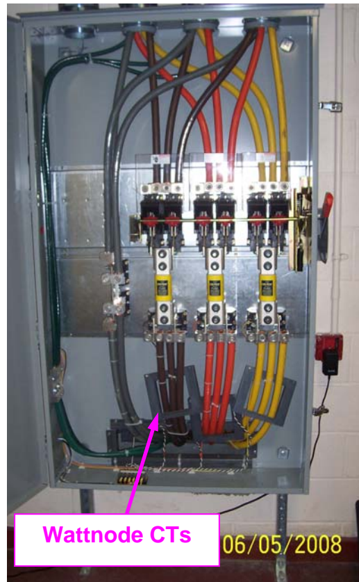
Generator Power CTs in Generator Disconnect
