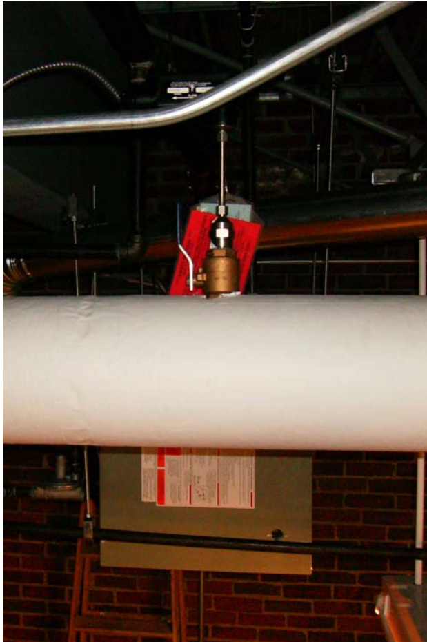
Loop Flow Meter (FL)
