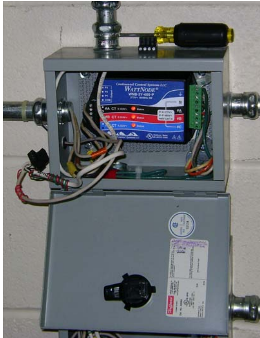
Facility Power Transducer (Yellow and Red LEDs for Negative Power with Low Power Factor)
