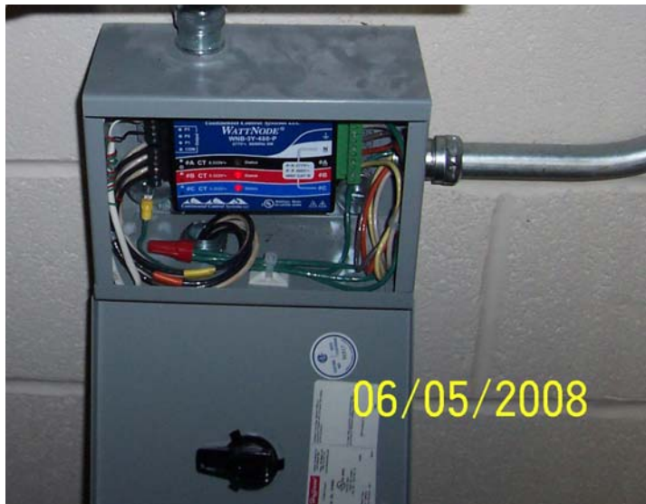
Generator Power Transducer (Red LEDs for Negative Power)
