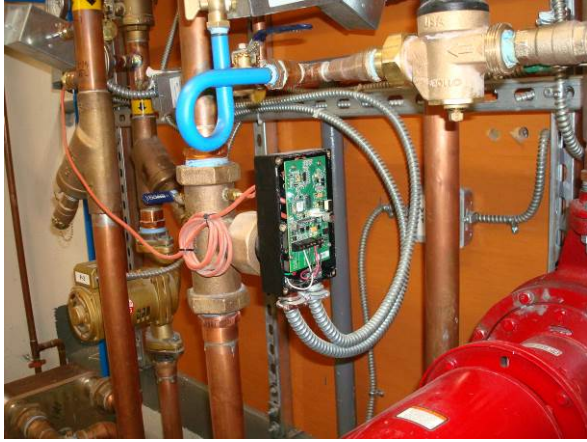
Badger 380 BTU meter (THW1, THW2, FHW).
