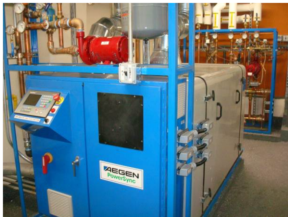
Aegen TP75-LE cogen unit located in basement mechanical room.
