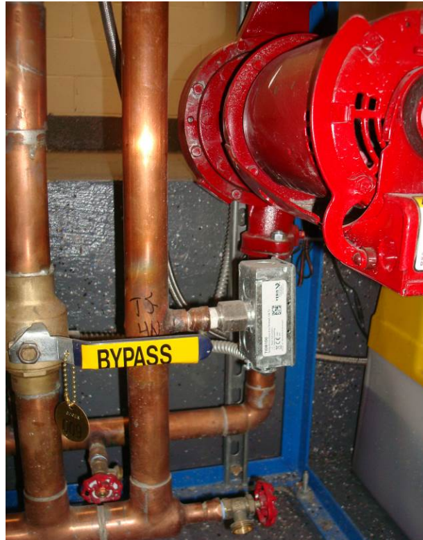
Mamac 10k Type 2 Thermistor (THW3), located in mechanical room.
