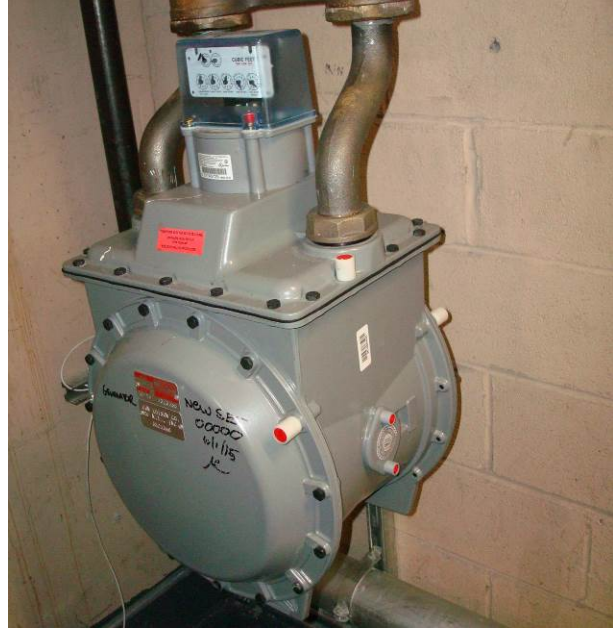
Con Edison cogen unit gas meter; awaiting pulse output.
