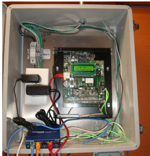
CDH panel containing data logger and CDH network switch.
