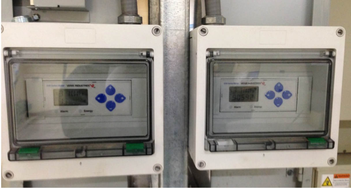
Power Meters (Measuring Power Output)
