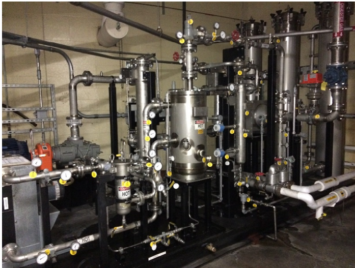
Gas Conditioning Skid
