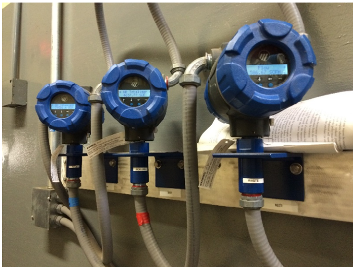
Gas Flow Monitors
