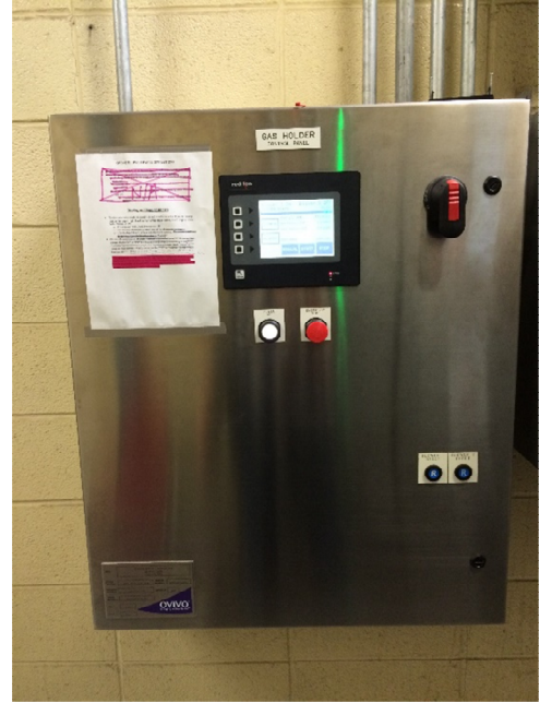
Gas Holder Control Panel
